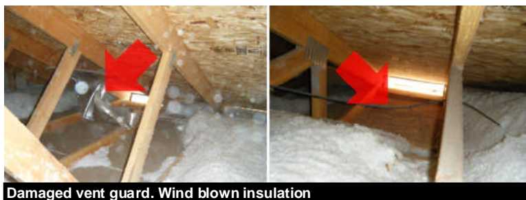
Damaged vent guard. Wind blown insulation
