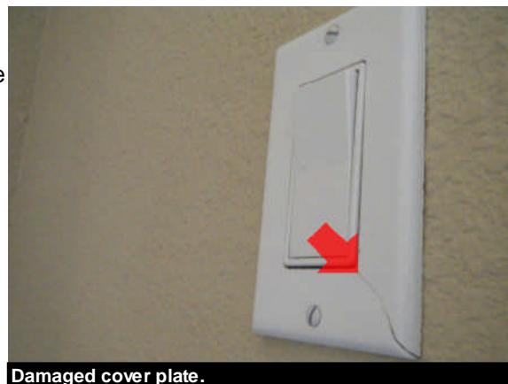
Damaged cover plate.
