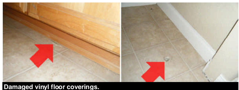
Damaged vinyl floor coverings.
