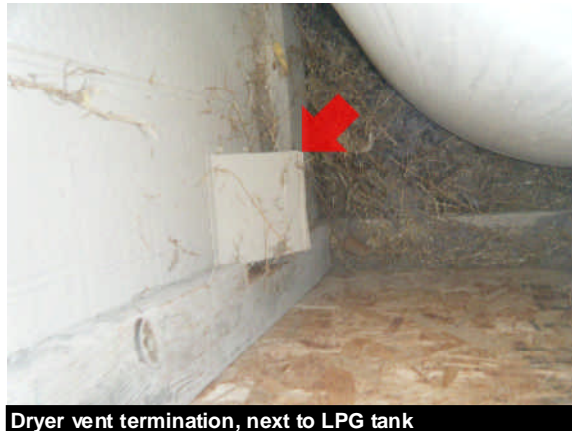
Dryer vent termination, next to LPG tank
