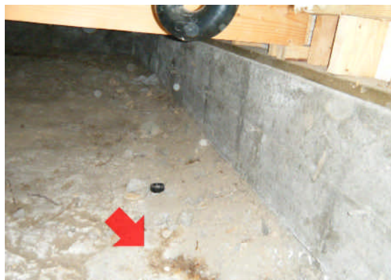
Signs of prior leaks in crawlspace.
