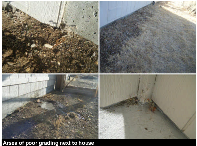
Arsea of poor grading next to house
