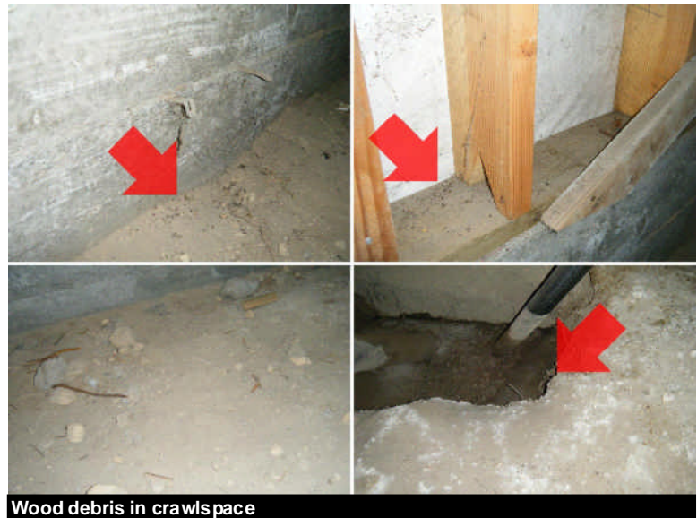
Wood debris in crawlspace
